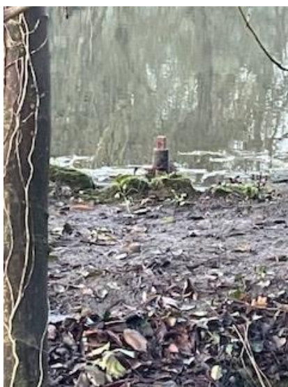
Figure 11: Photo of only sluice gate control at Denman College, Marcham (source Environment Agency)
